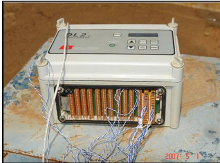
Figure 2 Data Logger to which thermocouples were connected
