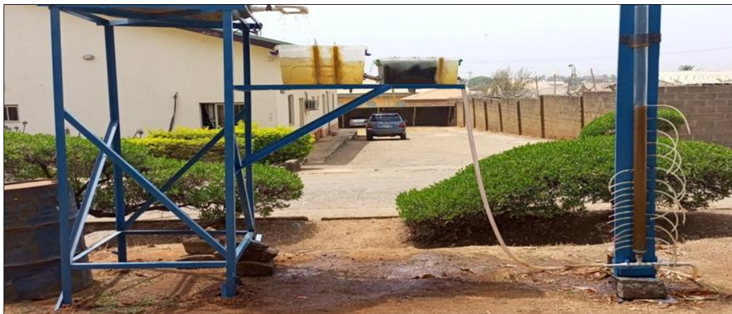
Figure 3 Photo of the constructed iron removal pilot model plant
